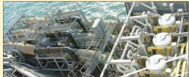
Figure 4.21 – Steam / seawater Vaporisers on Board the Excelsior .
