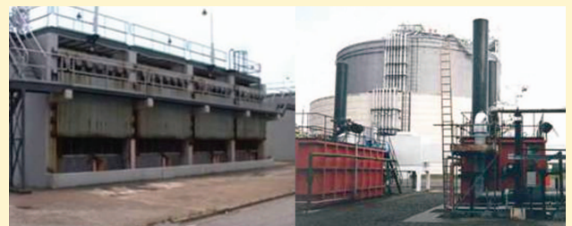
Figure 4.20 – Open Rack and Submerged Combustion Vaporisers.
